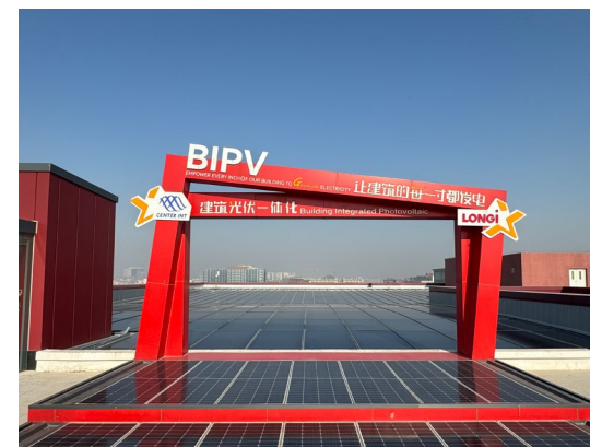
Rooftop PV System at Headquarters Office Building
