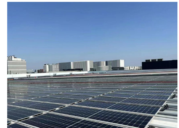
Rooftop PV System at Production Base
