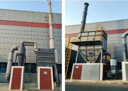
Waste Gas Treatment Equipment
